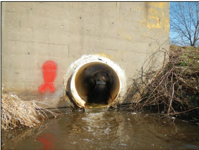
Figure 20: Road stream crossing on Gast Ditch at County Road 2 in Elkhart County. Note that the culvert is perched above the stream preventing fish from travelling upstream
